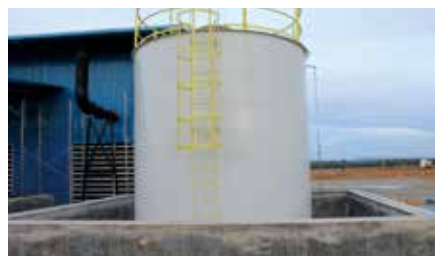
Leakage prevention sill around diesel tanks
