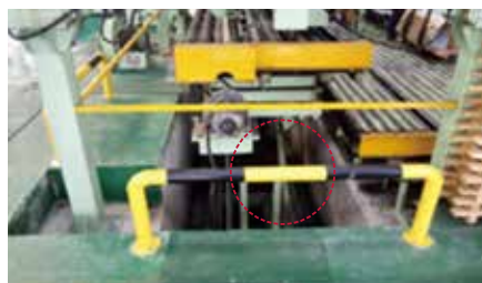
Safety bar installed at openings*
