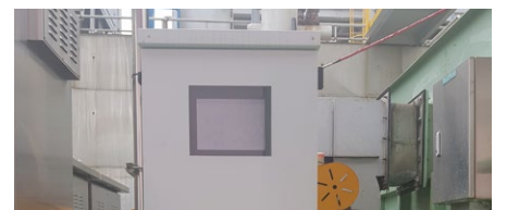
Odor monitoring facilities at the Ulsan Plant
