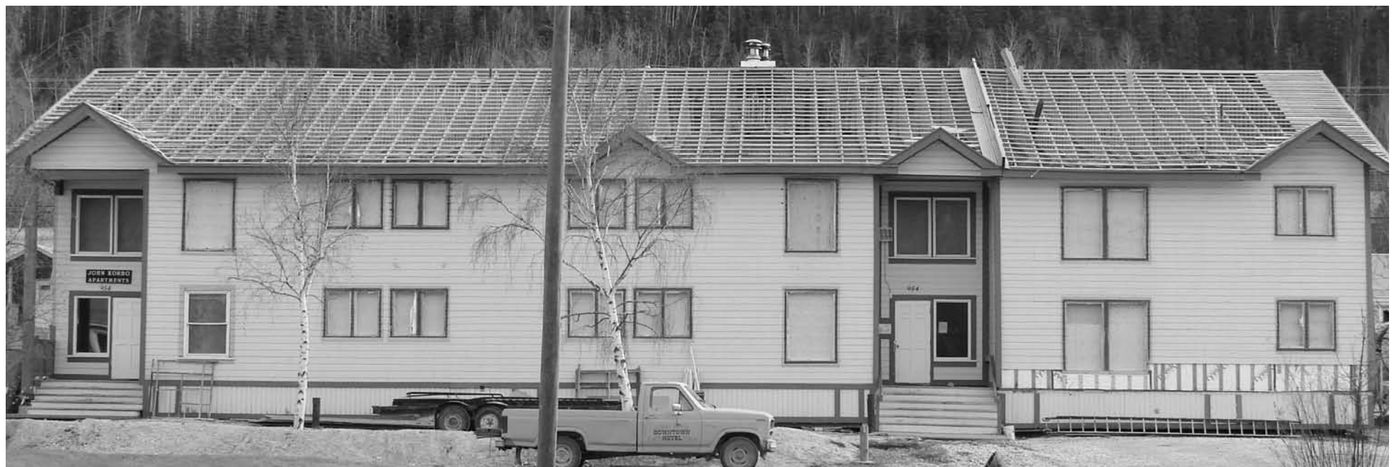
The roof and siding are coming off the decommissioned John Korbo apartments. There may be several layers to both as the building has been both retrofitted and given a new roof system within the last 20 years. Photo by Dan Davidson.
