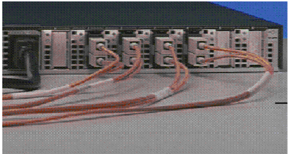
Figure 8. Fibre Channel Storage Hub
