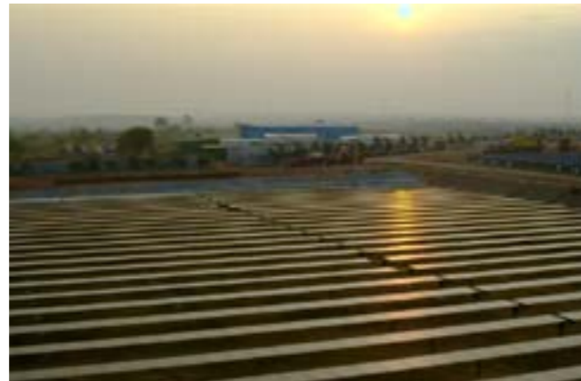
Solar plant in Sira, Karnataka
