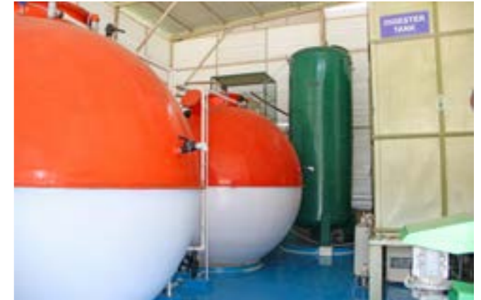
Biogas plant at an Infosys campus
