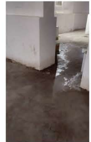
Water logging continues in basement of Cancer Hospital
