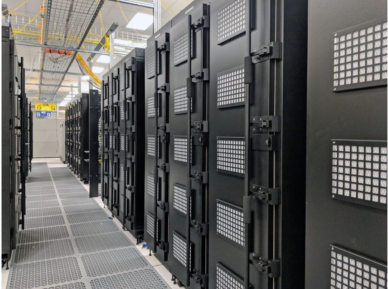
Fig. 15 - Electromagnetic pulse-resistant rack deployed in the Google production data centers.
