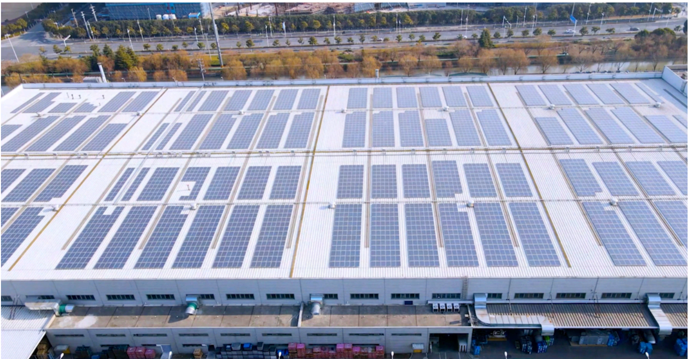
Solar panels in Taicang plant
