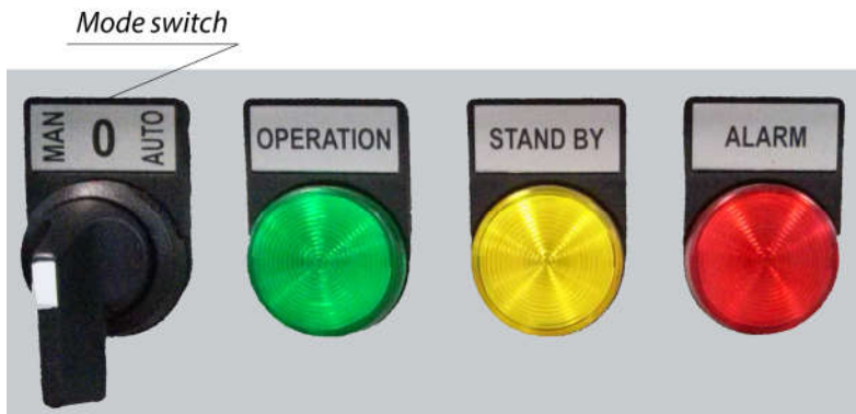
Figure 5.1: View of control panel
