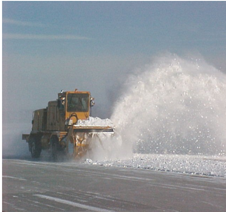
A sponsor's obligation to maintain the airport does not impose any specific responsibility to remove snow or slush or to sand icy pavements. To the extent possible, snow removal should be accomplished in those areas where public access is more likely. The sponsor, however, is responsible for providing a safe, usable facility. Where climatic conditions render the airport unsafe, the airport sponsor must promptly issue a Notice to Airmen (NOTAM). (Photo: FAA)
