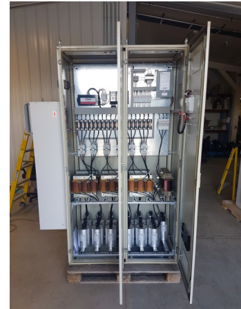
A 20+ year old Cos Phi power factor correction bank was sent in for refurbishing.
