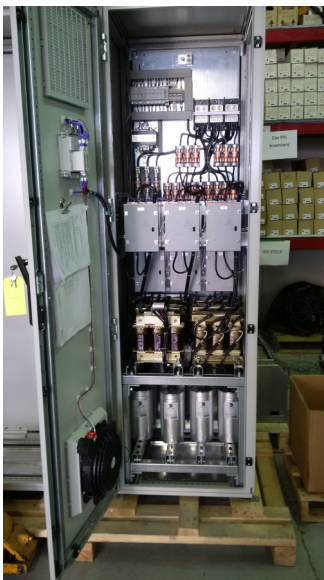
One of eight custom designed fast auto-switching power factor correction banks built and installed at Queens Park. (Ontario Government House)
