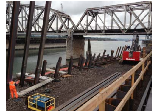
New soldier pile wall for retaining the hillside next to the new track area
