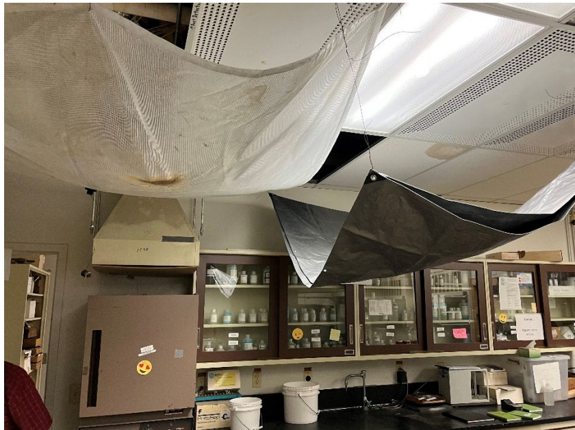
Figure 2 Tarps drain leaking rainwater into trash cans in Building 20 laboratories, trying to prevent damage to sensitive equipment.
