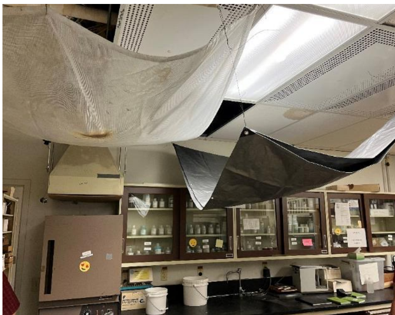
Figure 3 Tarps drain leaking rainwater into trash cans in Building 20 laboratories, trying to prevent damage to sensitive equipment
