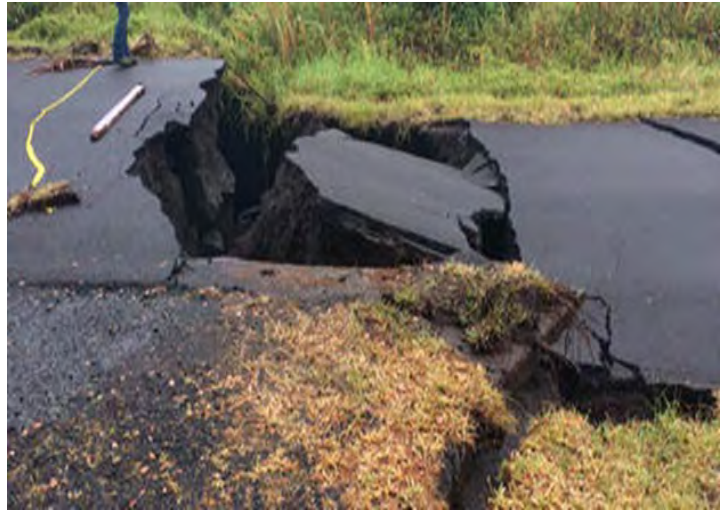
During an earthquake, a surface fault cracked and ruptured an asphalt road surface. Source: USGS.
