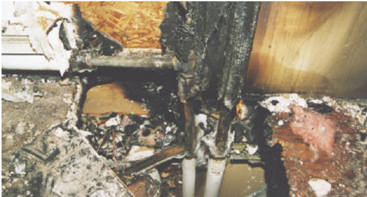
Figure A1: Fire origin traced back to hot-water pipes in bare-contact with a floor assembly [46]
