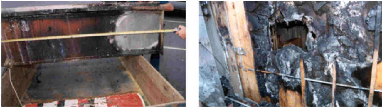
Figure A2: Heating pattern on back of ‘cheese-melter’ and corresponding burn pattern inside the wall assembly [47]
