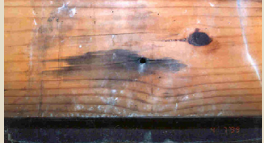
Figure A3: Charring occurring around a screw mount after long-term installation of an industrial ‘cheese-melter’ [47]
