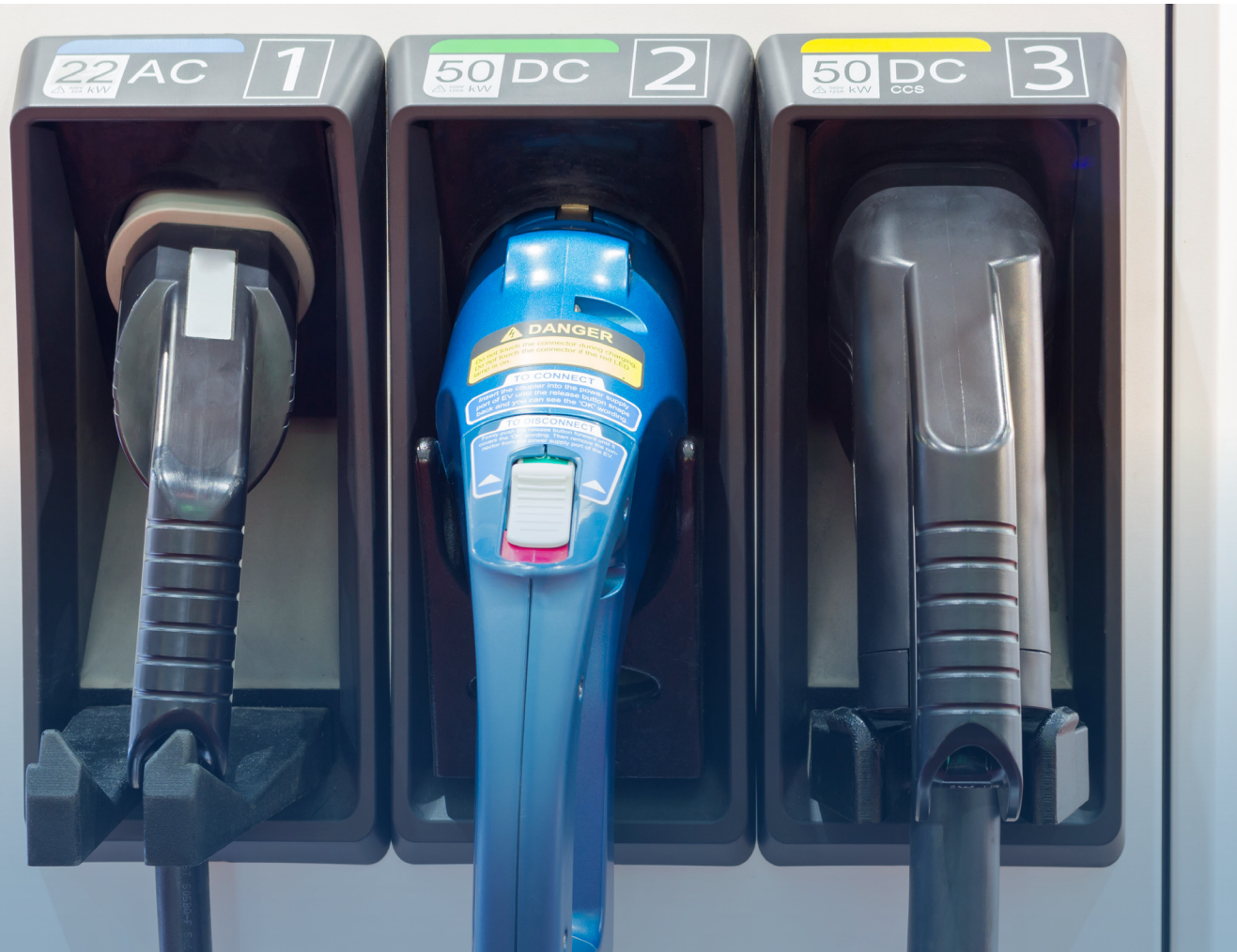
Figure 12 – DC Fast Charger
