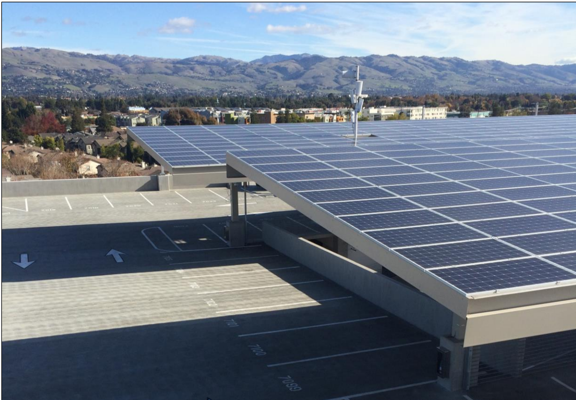
FIGURE 2: SOLAR PV PANELS ON BART BERRYESSA PARKING GARGAGE
