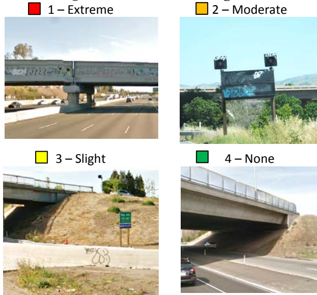
Figure 26. Graffiti Grading Scale.
