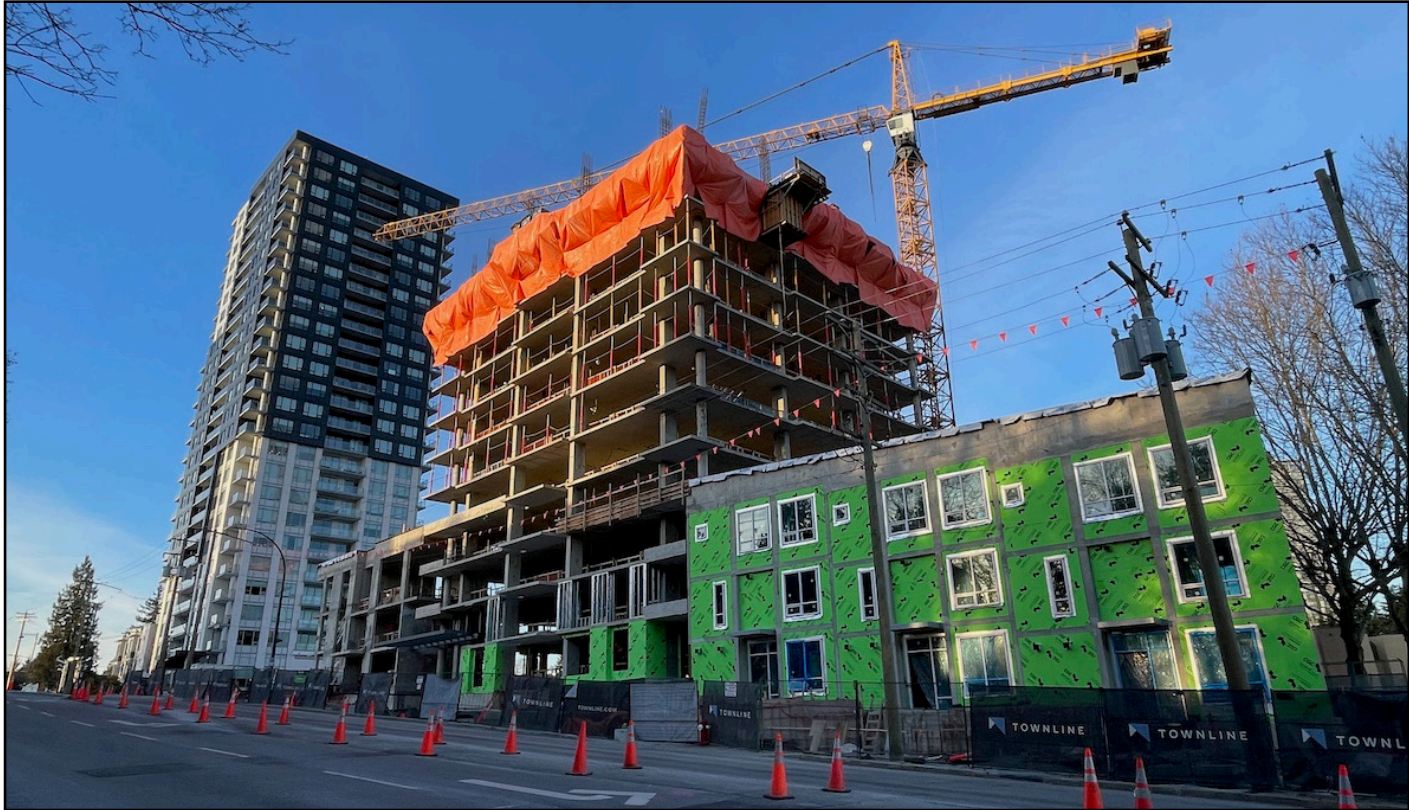
The Holland Two - Phase 2 of Townline's Holland beginning to rise above Old Yale Rd
