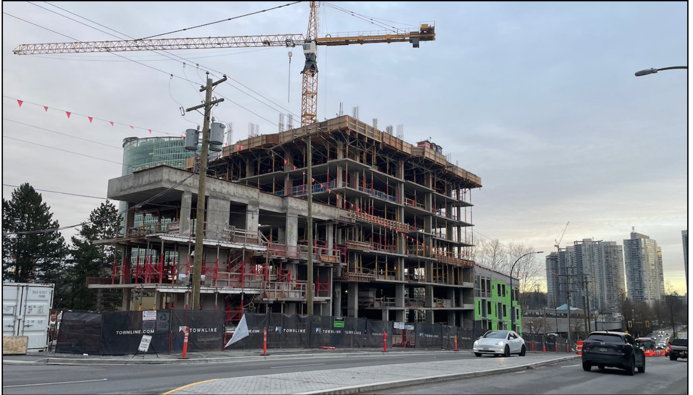
The Holland Two - Tower beginning to rise above podium along Old Yale Rd
