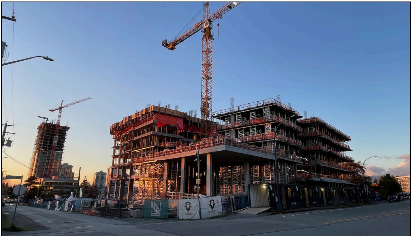
Flamingo One - 6-Storey office podium taking shape along Whalley Blvd with residential tower rising above
