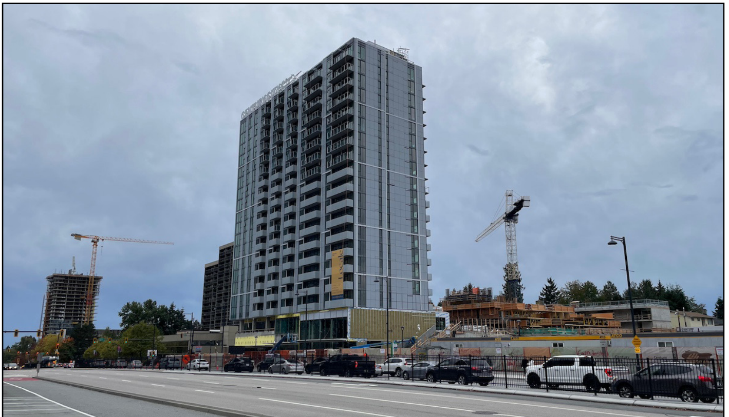
Century City Holland Park - First market residential tower beginning to rise behind rental tower
