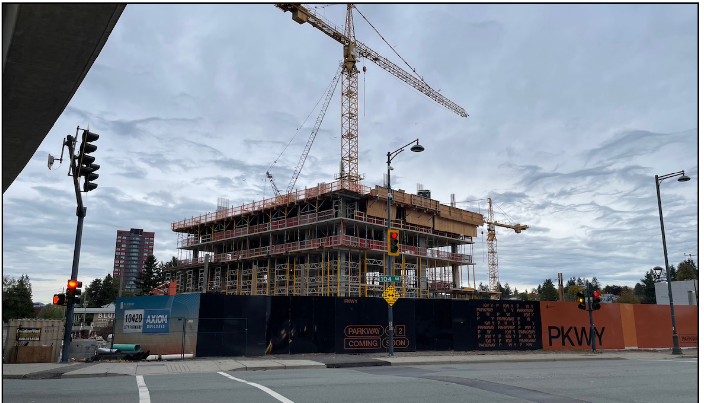
Parkway - First tower beginning to rise at corner of 104 Ave & City Parkway
