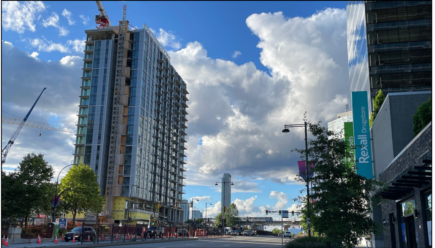
Century City - Rental tower nearing completion with market tower phases proceeding behind
