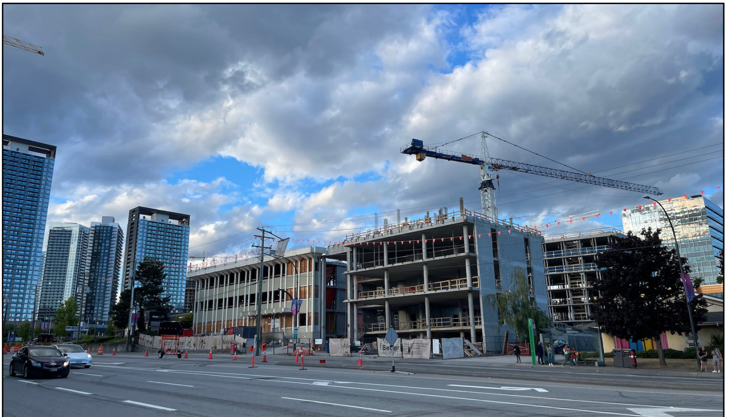
Comma King George - Office podium taking shape with residential tower beginning to rise behind
