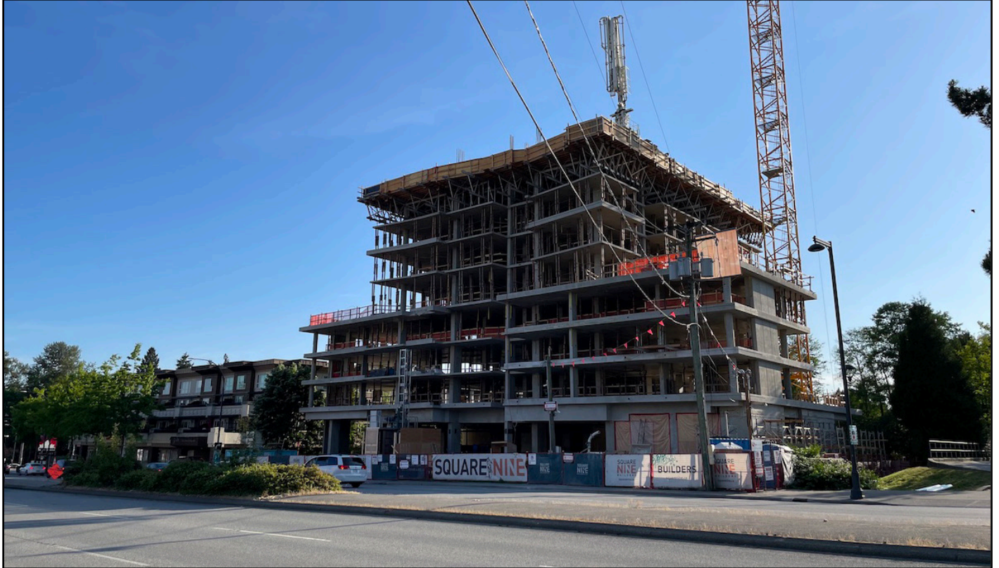
Belvedere - Tower beginning to rise above podium along King George Blvd near 96 Ave
