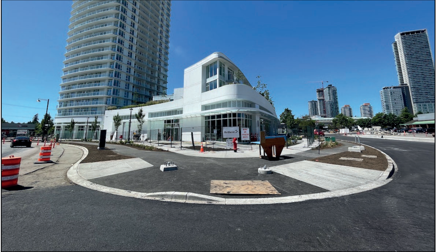
Georgetown One - New curb, sidewalks, and bike lanes now installed along Whalley Blvd and 102A Ave
