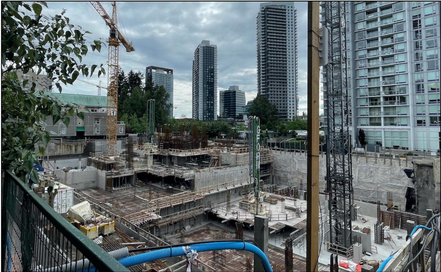
Park George - Parking levels construction continues / now at grade for rear portion of site
