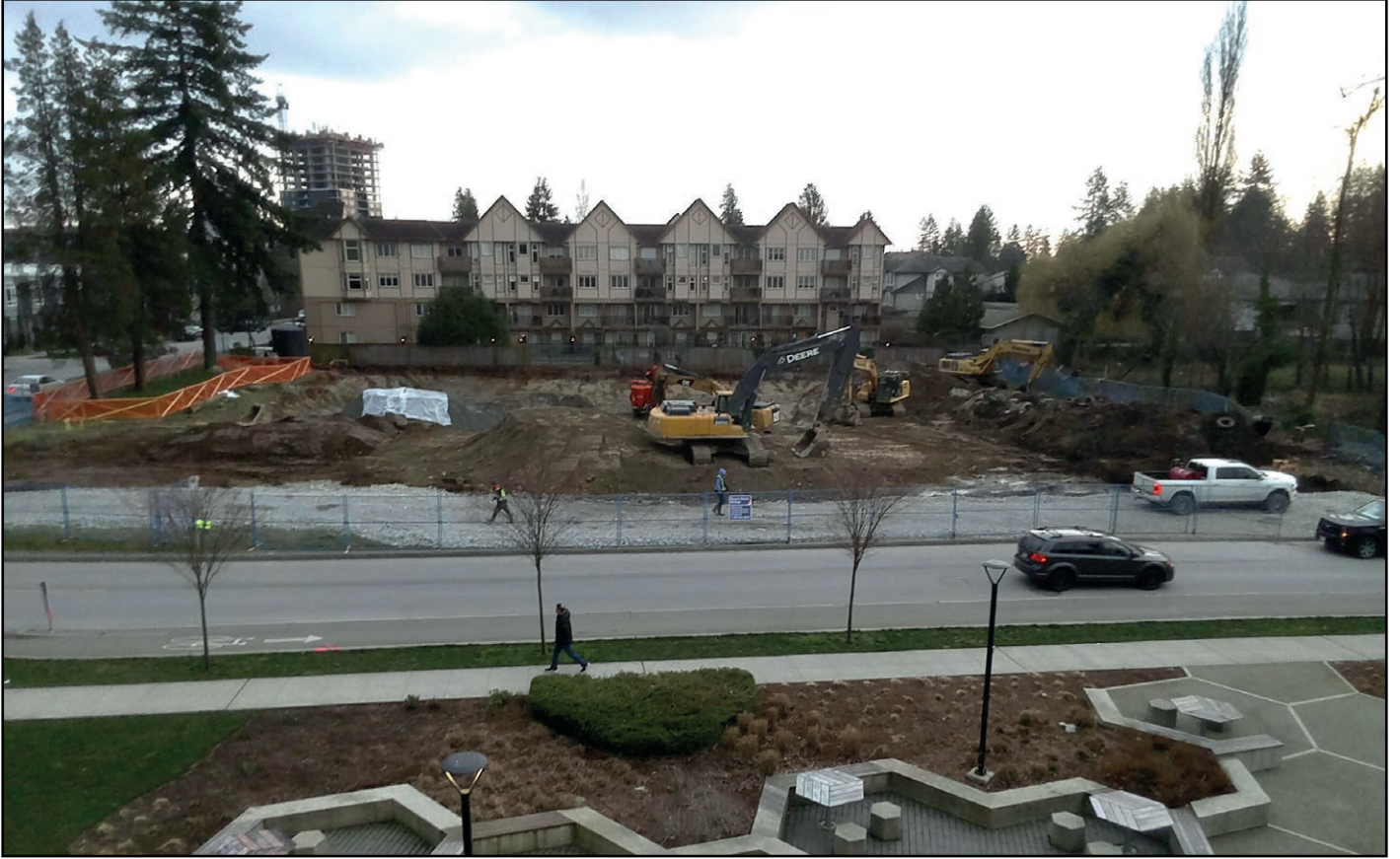
Melrose - Site clearing & excavation now underway for this 26-storey tower by ML Emporio located at 133 St & Central Ave across from West Village Park.
