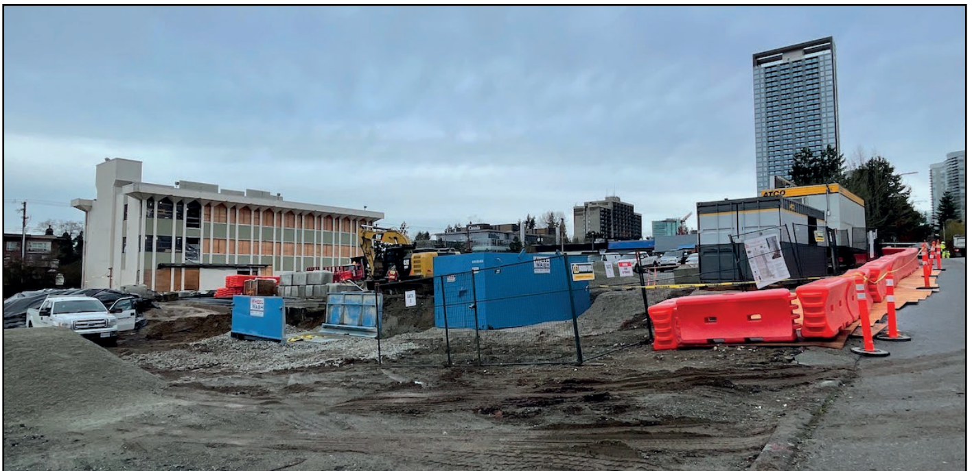
Parks & Yards (38-Storey Residential, Office, Retail) - Site preparation and heritage building restoration now underway
