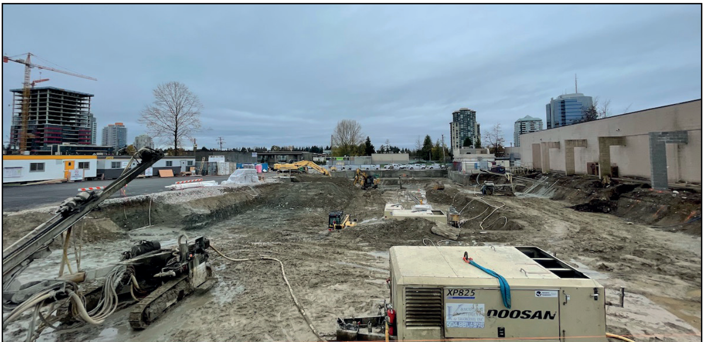
The Grand - Excavation has begun for The Grand on King George (46-storey condominium above a 5-storey office & retail podium)
