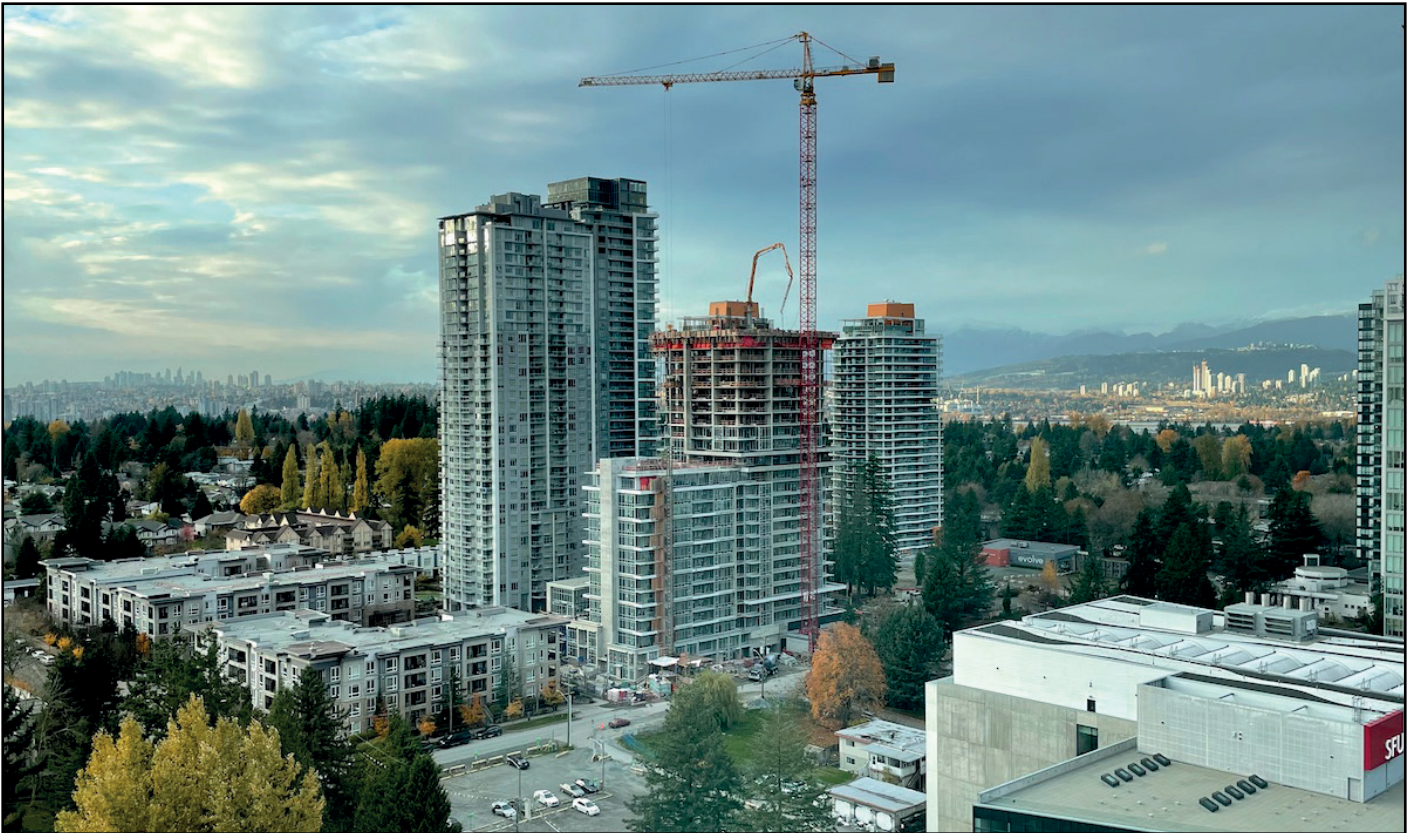
One Central - Tower continuing to rise above podium with 20 levels remaining before reaching a final height of 44-storays
