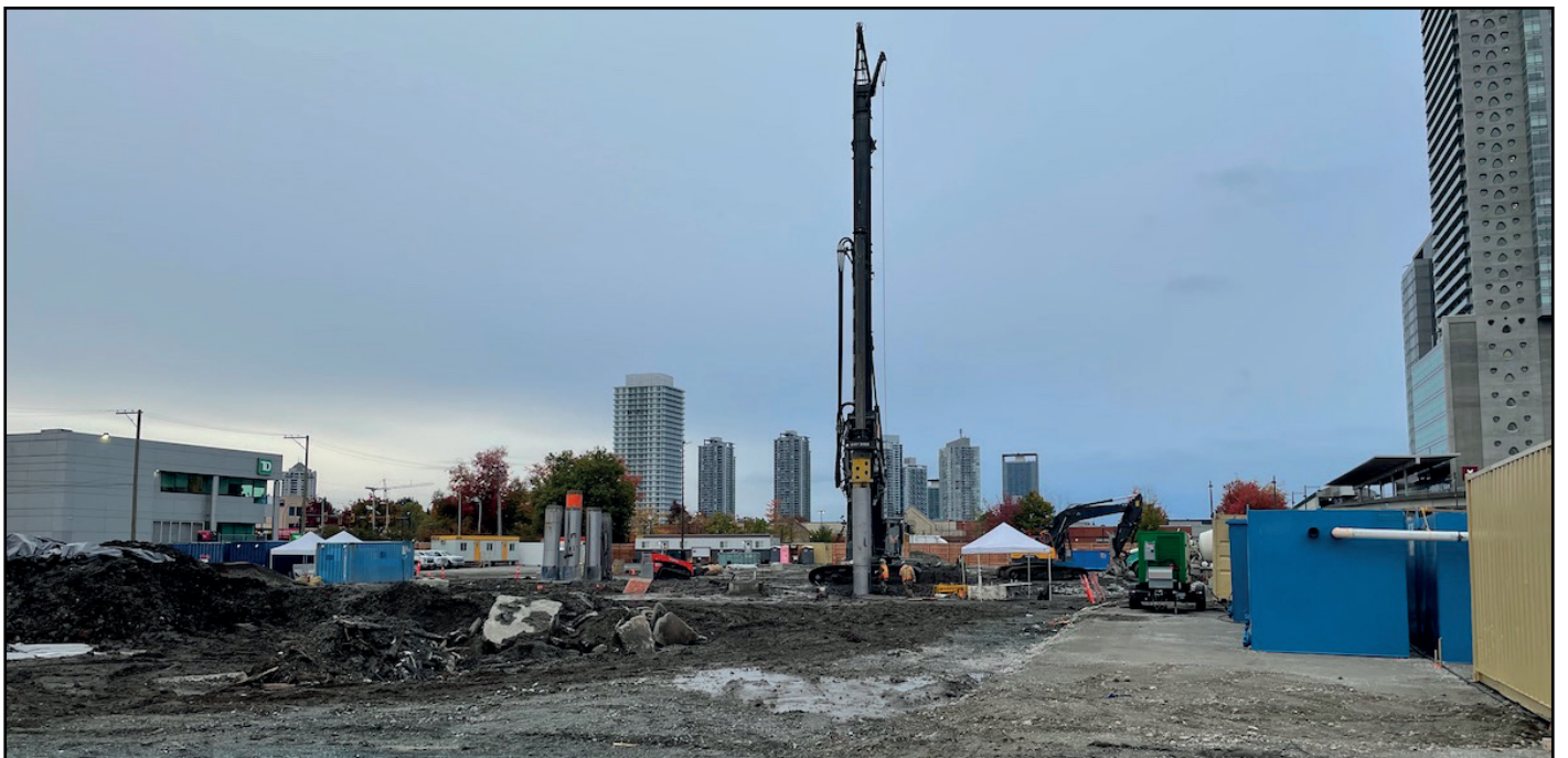
Brightside (Phase 1) - Site preparation and drilling underway for Phase 1 (38-storey rental tower with ground level retail)
