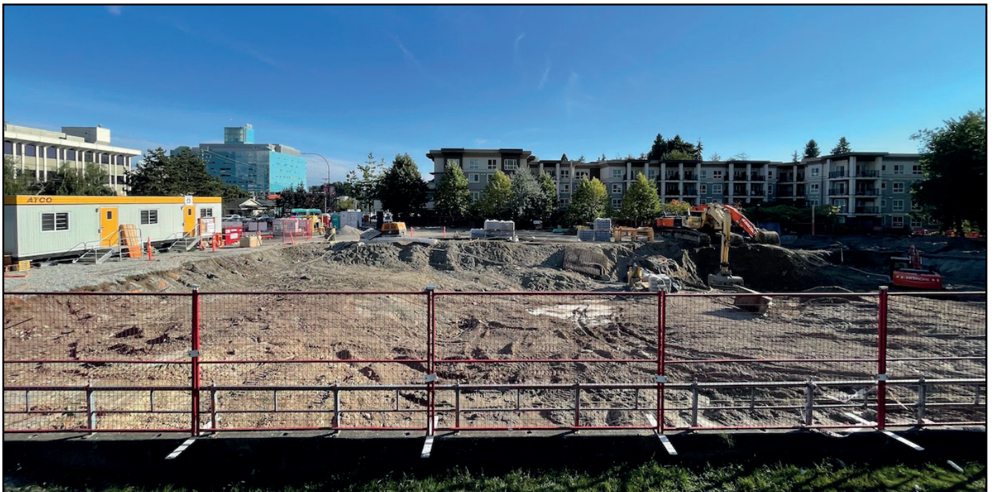
Belvedere - Excavation now underway on this 27-storey residential tower, with ground level retail
