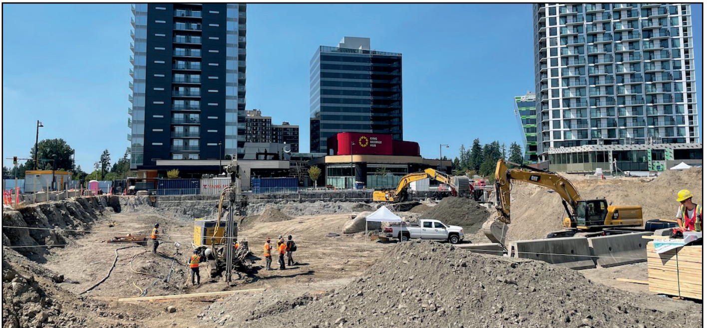
Plaza One & Two @ King George Hub - Excavation now underway for the final phase of King George Hub
