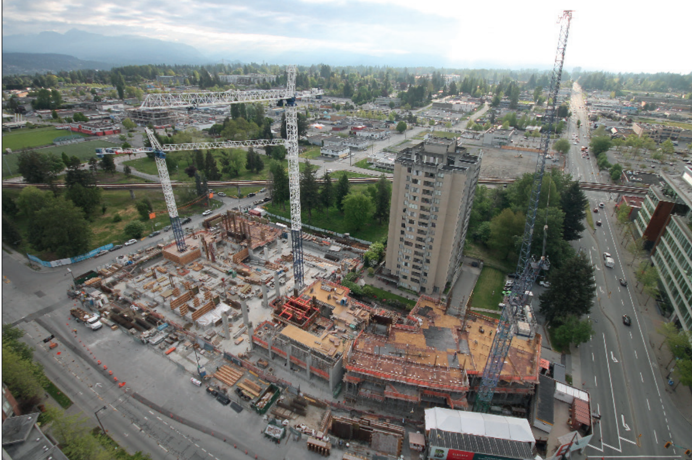
BlueSky's University District beginning to rise above ground at 104 Ave & University Dr
