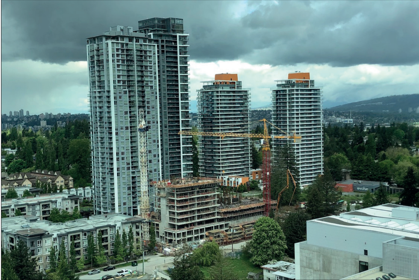
One Central's podium (left) rising to its ultimate 13-Storey height, with the main tower (right) following behind
