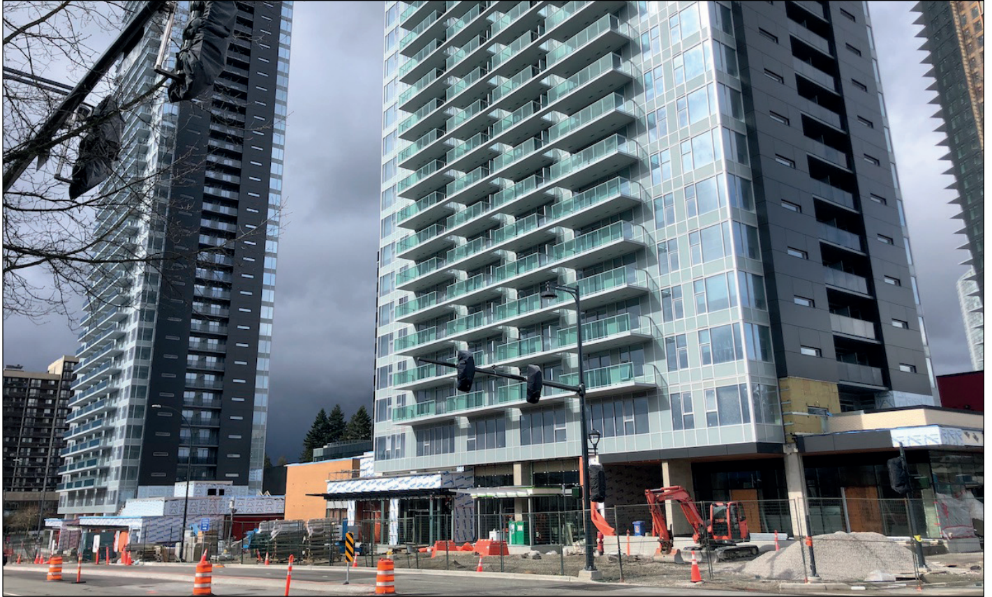
King George Hub residential towers and retail nearing completion along Fraser Highway
