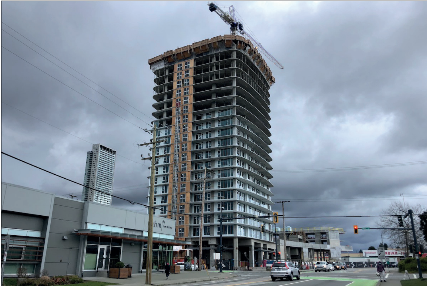
Georgetown One by Anthem beginning to transform the corner of 102 Ave & Whalley Blvd
