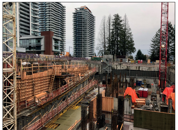
One Central | 44-Storey Residential + Retail
