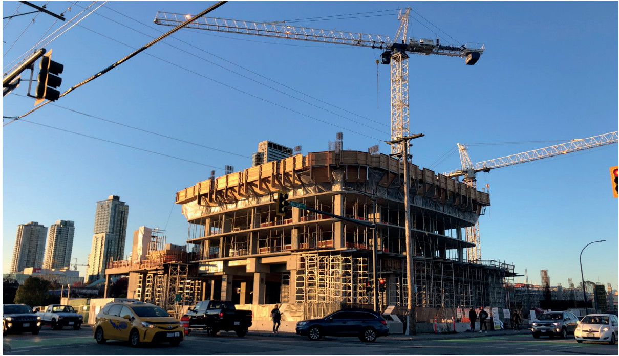
Georgetown One | 30-Storey Residential + Retail
