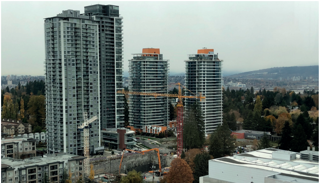
West Village Construction: One Central (44-Storey Residential, Retail) in forefront; Linea (28-Storey Residential) far right.
