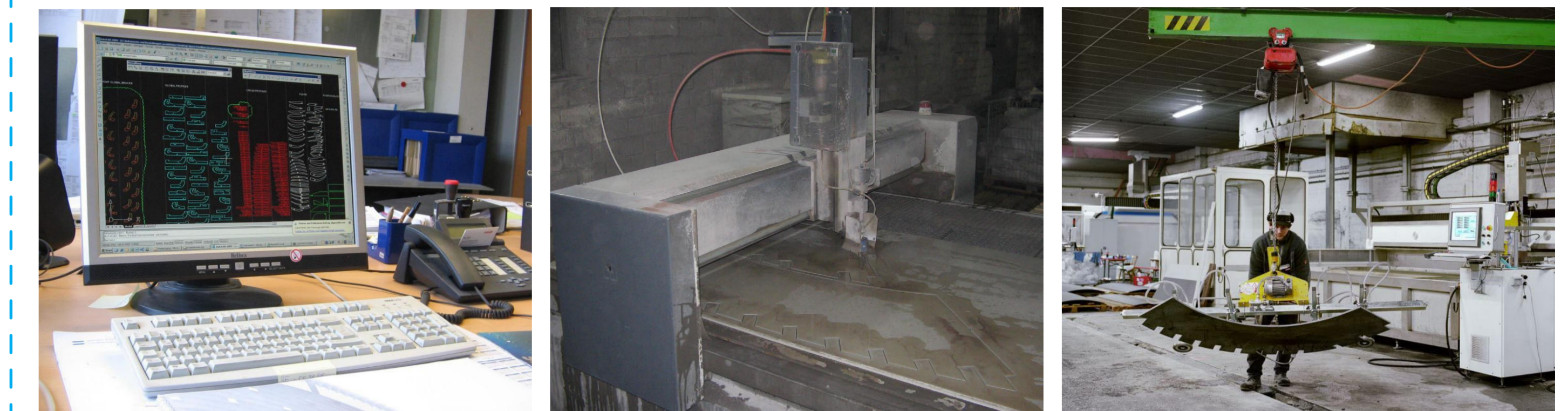
Individual fibreC elements were manufactured off-site using water jet machine. The material for the primary ribs has a thickness of 13mm, while the material for the secondary profiles was 10mm thick to reduce the self-load of the pavilion.
